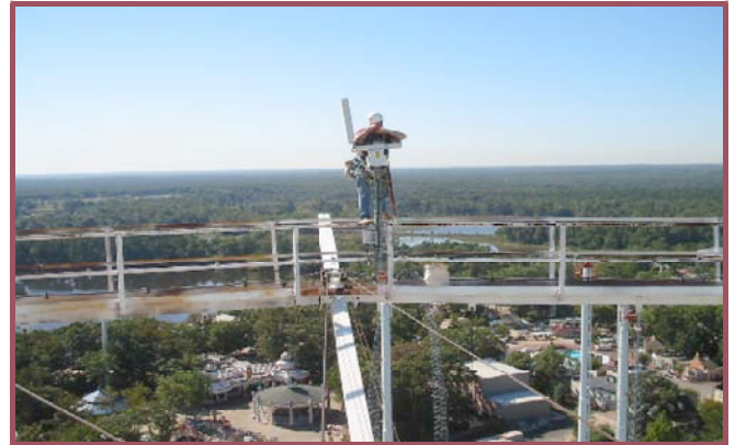
DSI Project Manager performing maintenance on the camera system
