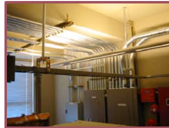
Completed electrical installation
